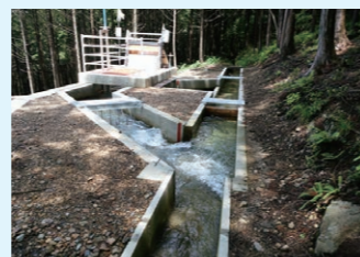
Ochiai Hiraishi small-scale hydroelectric power station (Gifu Prefecture)
