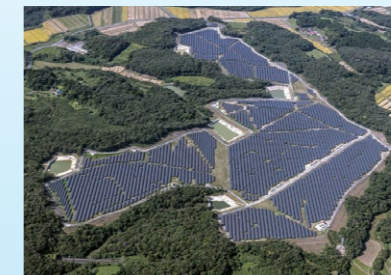
Mega Solar Park (2020) To make the most of renewable energy and to achieve carbon neutrality, we installed 122,000 solar panels on a vast 65 ha site developed as part of a mega solar power plant project with an output power of 45 MW in Miyagi Prefecture.
