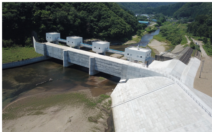
Disaster restoration work at Tashiro River sluice gate and surrounding area [Iwate]
